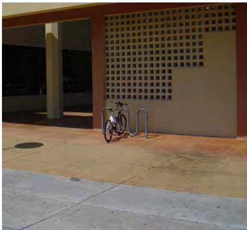
Bike Rack Installed Too Close to a Building, Which Limits Appropriate Use of the Rack
