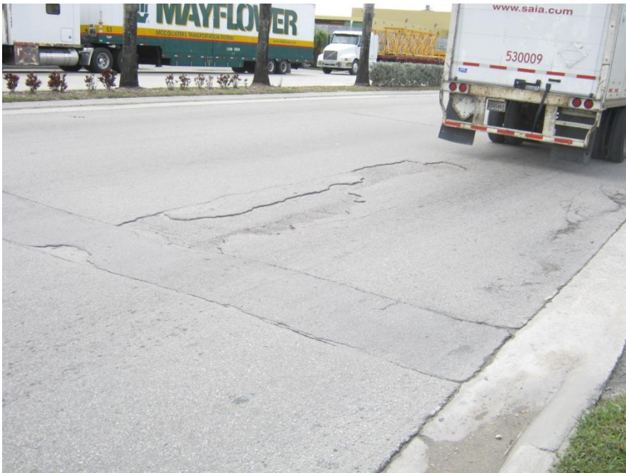
Eastbound NW 116 th Way east of NW South River Drive - Poor pavement conditions
