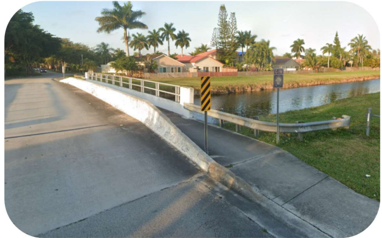
Bike/ped crossing to be utilized for the Black Creek Trail across canal C-1W on SW 155 th Avenue. Image Source: Google Street View, 2022 .
