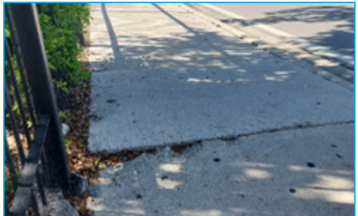
Uneven sidewalk along Miami Lakes Drive creates potential trip hazard
