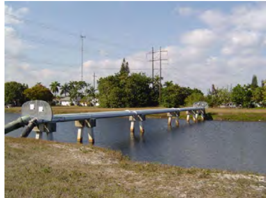
Low Pipeline Crossing the Snake Creek (C-9) Canal
