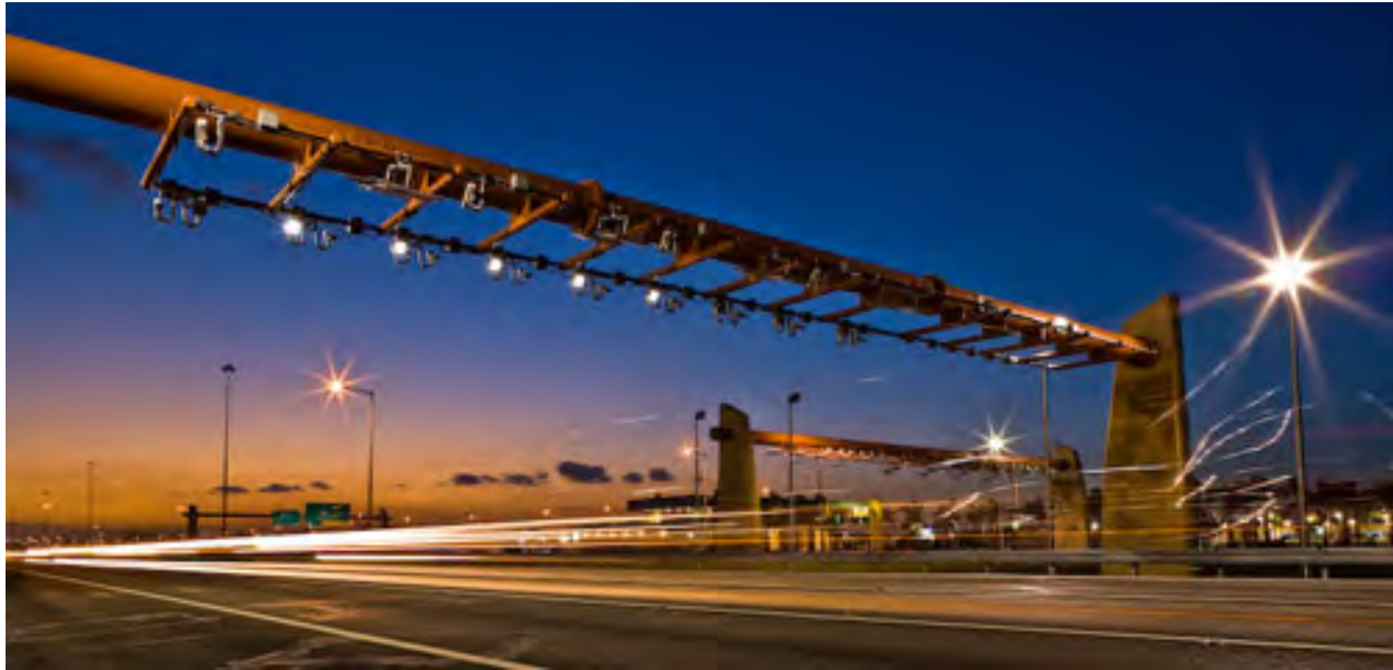
Open-Road Tolling Gantry, Miami-Dade Expressway (MDX) Facility
