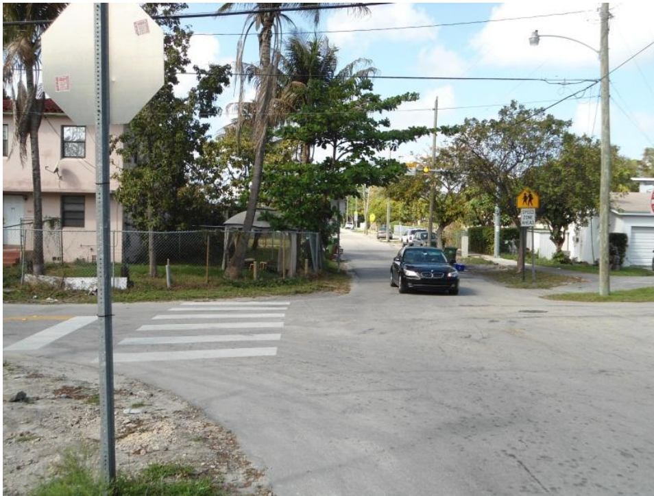
Crosswalk without access ramps and paved sidewalks
