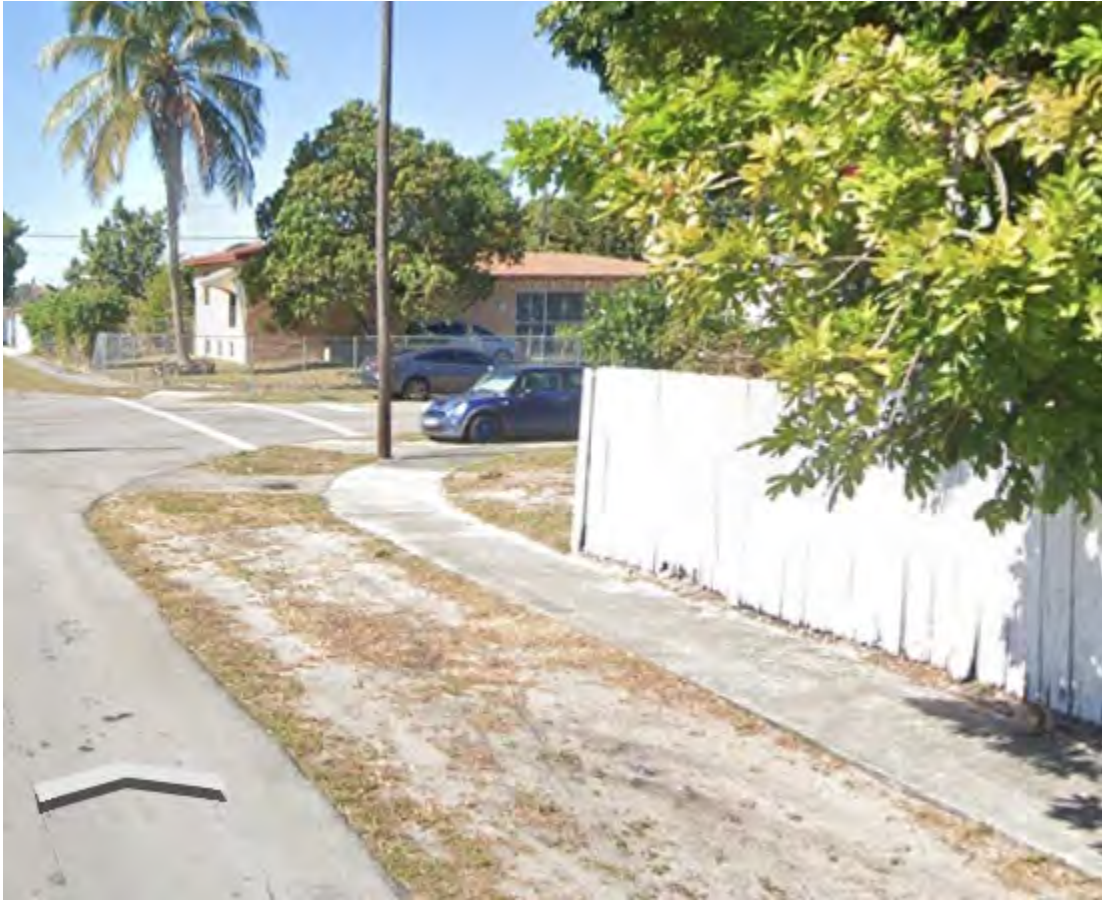
21. Repair sidewalk, Poses Tripping Hazard
