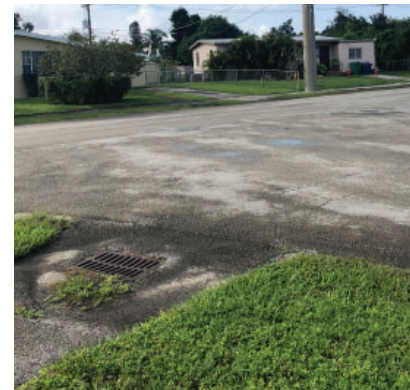
Missing ADA Features
