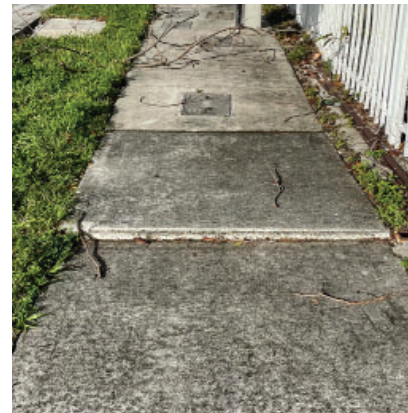
Damaged / Settled Sidewalk
