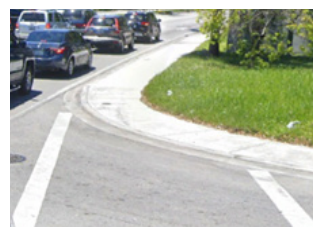
Missing detectable warning surfaces
