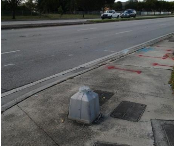
Pedestrian Push Button Pole Missing
