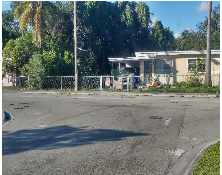
Faded pavements markings
