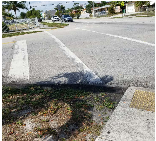
Faded pavement markings
