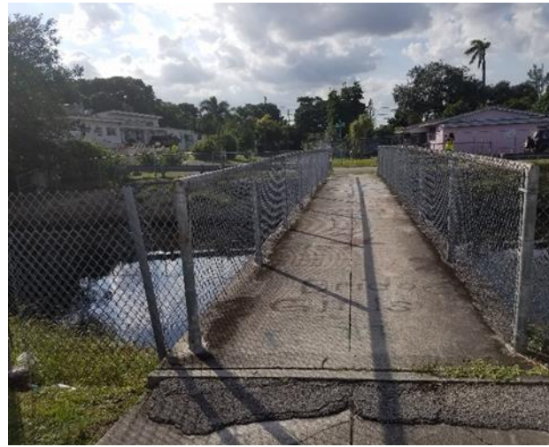
Figure 60: Bridge Maintenance Required
