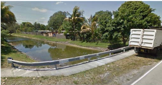
Missing pedestrian railing along canal
