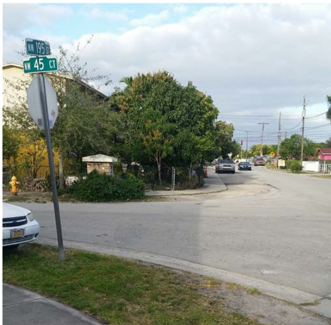
Missing curb ramps and pavement markings
