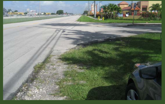
Unpaved sidewalk along a potential pedestrian route to Hialeah Gardens Elementary
