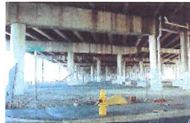
Horrific conditions beneath I-395
