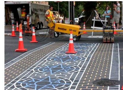
Painted/textured crosswalks can be achieved through the application of thermoplastic striping, and applied to raised crosswalks as well.
