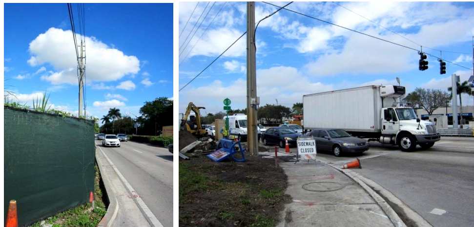
(L) Construction fence eliminates possible pedestrian pathway on NW 58 th Street. (R) Though the sidewalk is closed, the expanse of the construction makes it difficult to determine an appropriate detour route. The lack of a crosswalk also complicates matters here on NW 25 th Street.
