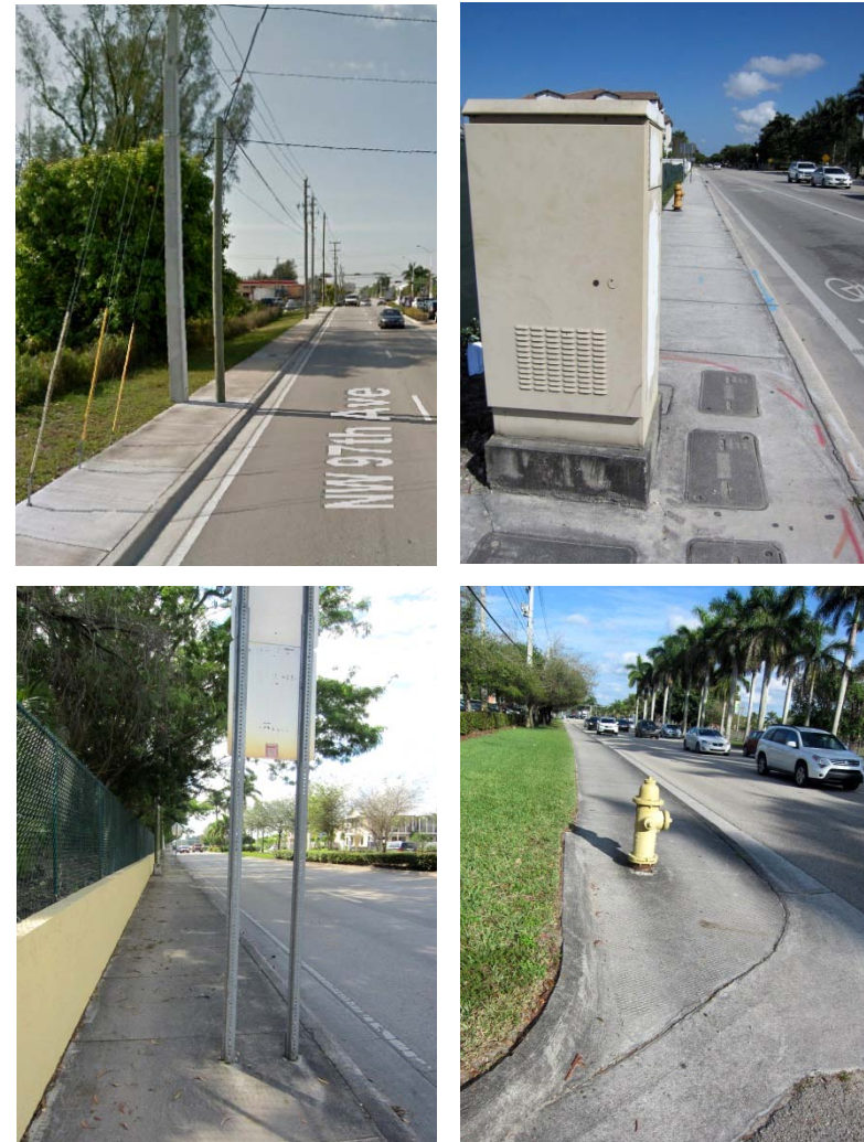
Observed sidewalk obstructions include utility poles in the middle of the sidewalk, with additional cables blocking the path for an alternate route (Top Left, Image source – Google Earth), Utility boxes and fire hydrants in sidewalks (Top Right), traffic signs (Bottom Left), and fire hydrants in sidewalks at curb areas (Bottom Right), all of which present issues for pedestrians, and some of which are non ADA compliant.
