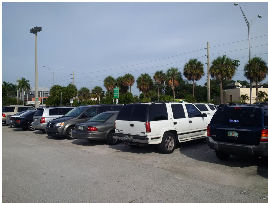
Faded pavement markings
