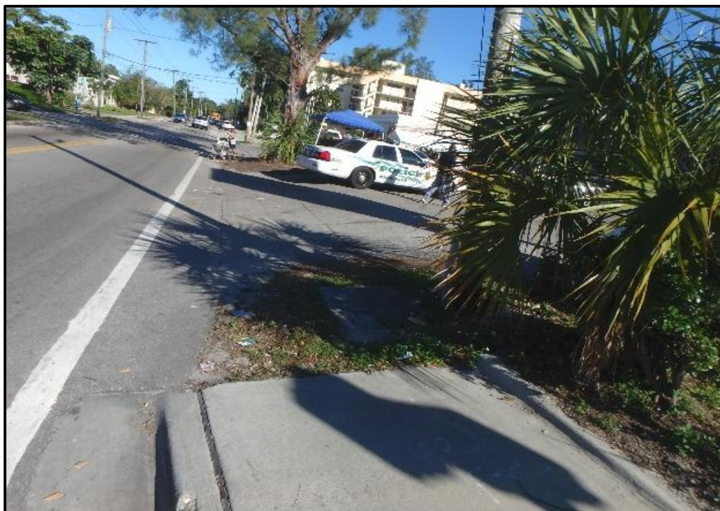
Photograph 8: Sidewalk discontinuity on the south side of east leg
