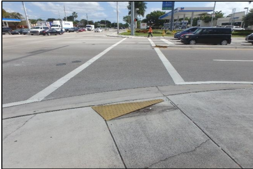
Photograph 17: Damaged pedestrian detectable warning mat at southwest corner
