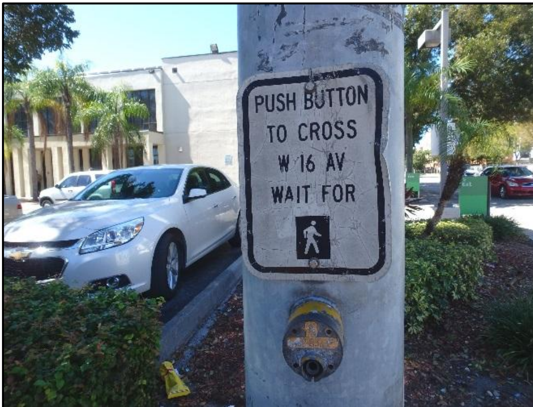
Photograph 28: Damaged push button and sign panel at southwest corner
