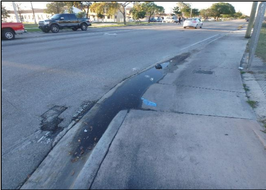
Photograph 14: Water ponding at northeast corner of NW 12 Avenue intersection
