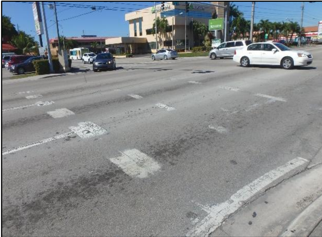
Photograph 26: Faded crosswalk markings
