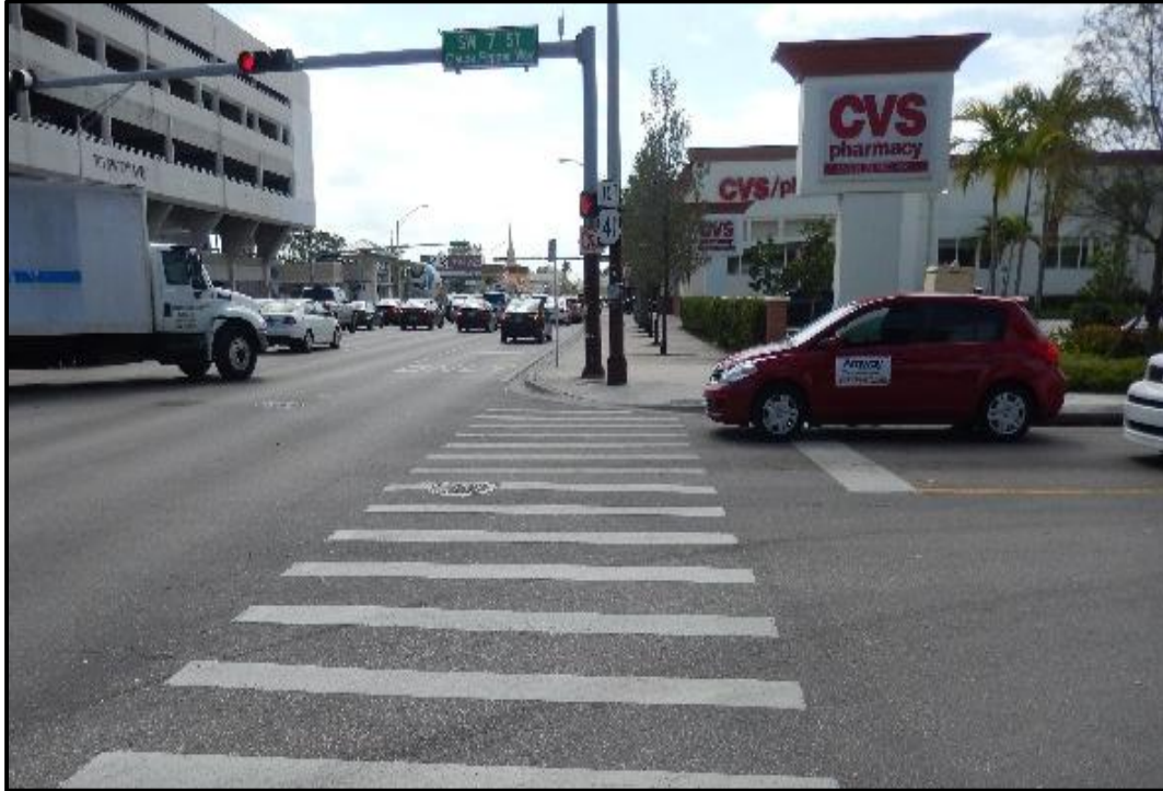
Photograph 4: Missing pedestrian crossing signage at the southwest corner
