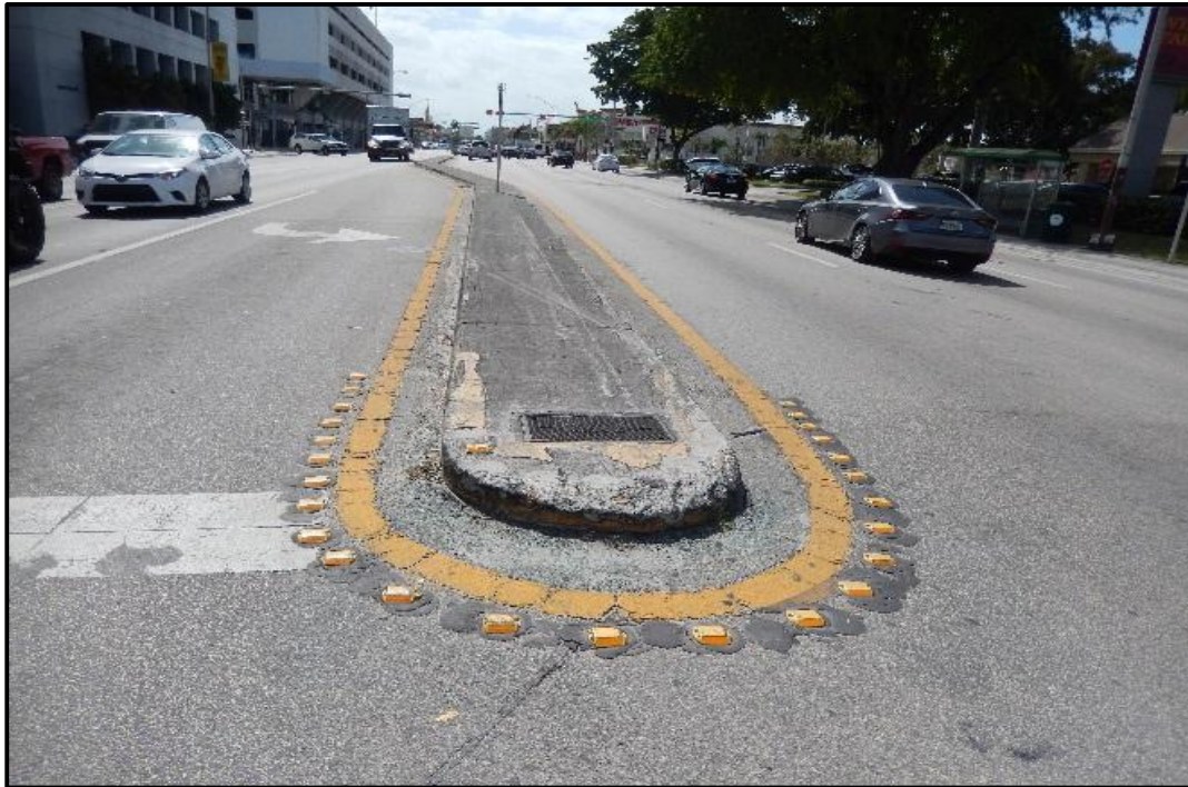
Photograph 2: Traffic separator damaged by traffic
