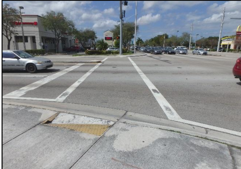
Photograph 16: Damaged pedestrian detectable warning mat at southeast corner
