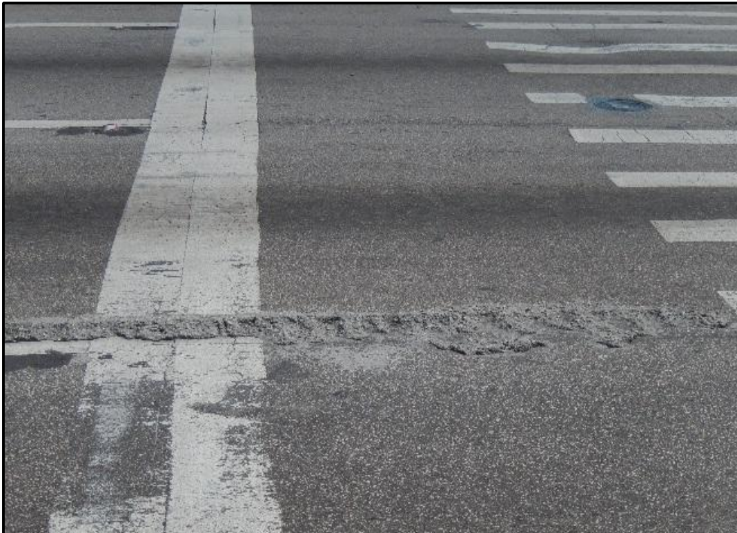
Photograph 3: Large ridge of cement along the SB lanes and leading into the crosswalk
