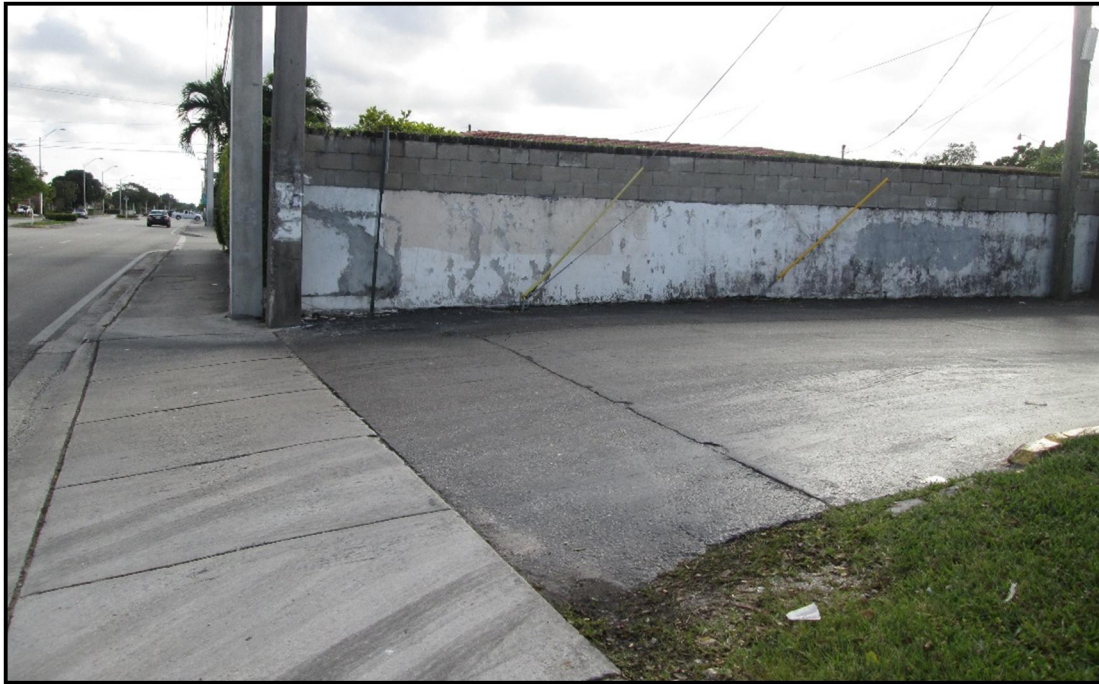
Photograph 46: Privacy wall on the west side of SW 87 th Avenue/south leg (looking south)
