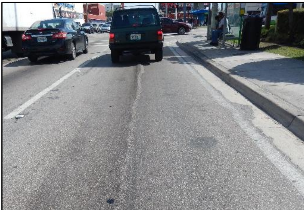
Photograph 11: Uneven pavement on eastbound outside lane
