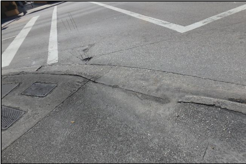
Photograph 27: Pedestrian ramp at northwest corner not ADA compliant
