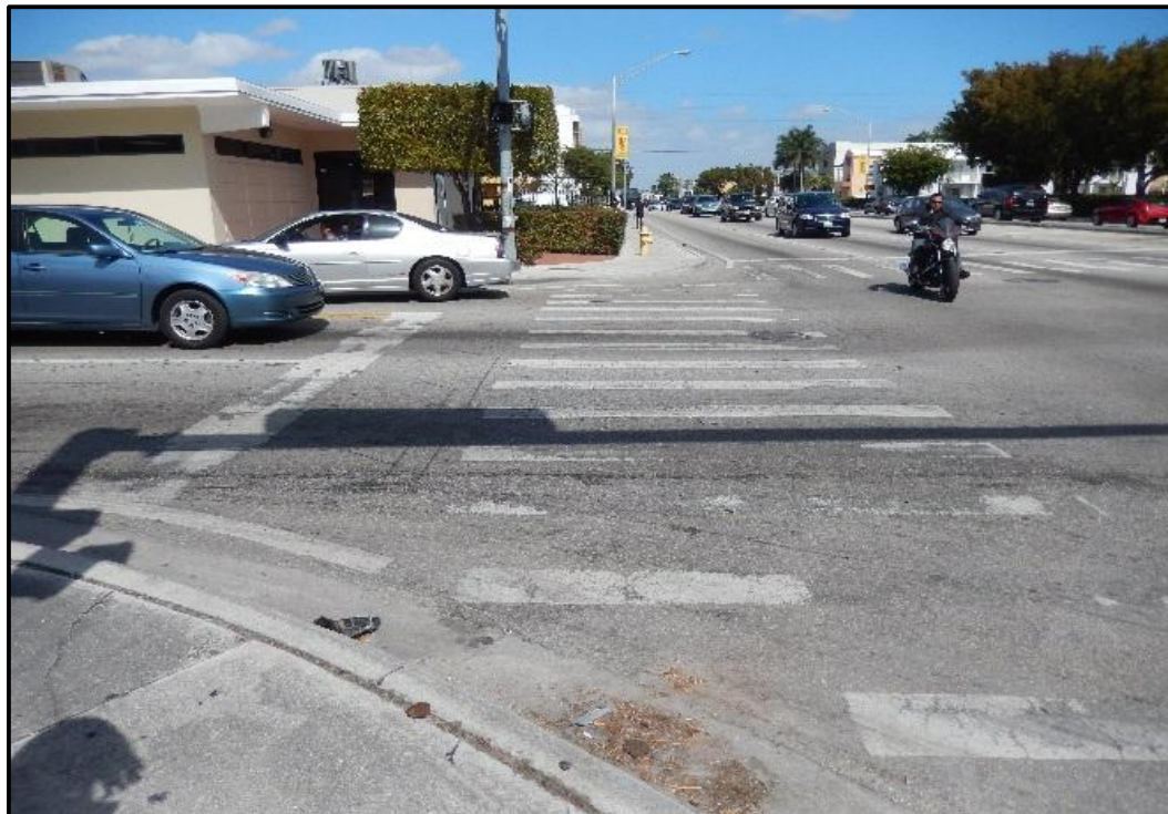
Photograph 1: Worn out pavement markings
