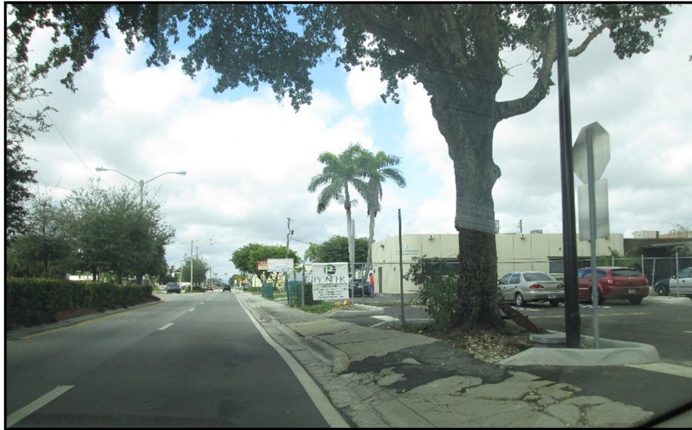
Photograph 55: Broken sidewalk near Washington Avenue
