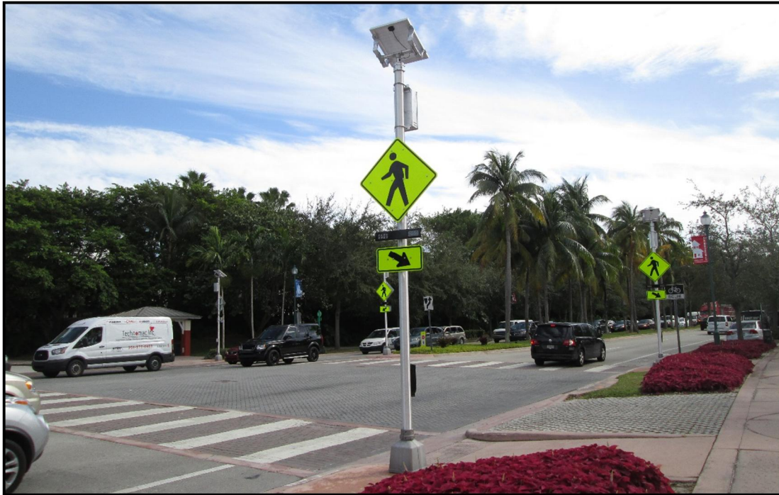
Photograph 31: RRFB at Heather Drive
